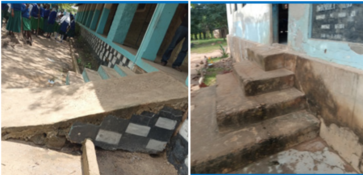
Field Photo: Showing stair case with ramps for ease of access(left), and stair case without ramps (right)
